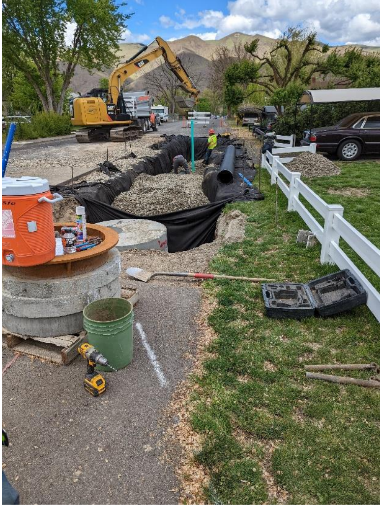
Figure 39: Installation of infiltration trenches in Clarkson, Washington. Installation of infiltration trenches in Clarkson, Washington.
