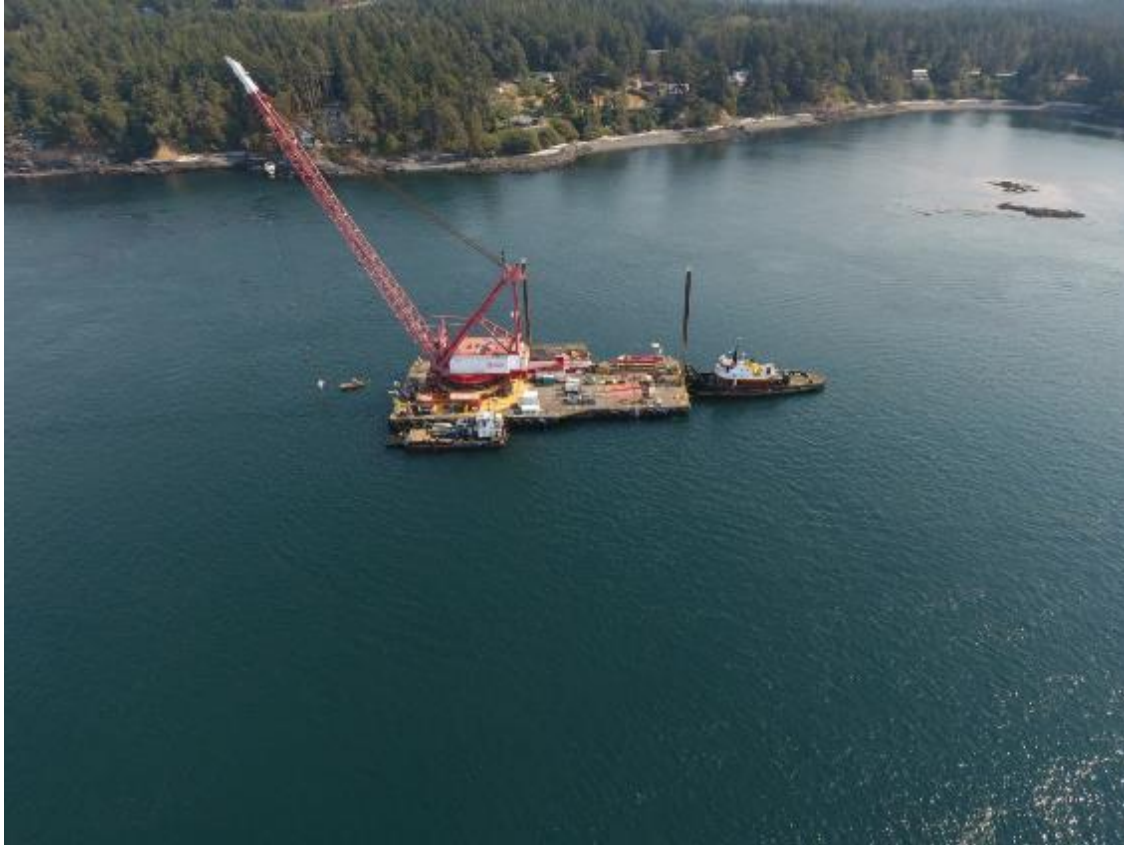
Figure 36: Tug, barge and crane on site, August 2023, San Juan County. Credit: Ecology
