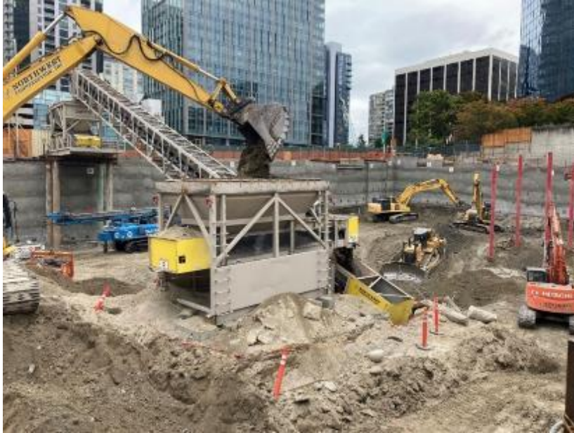
Figure 33: CID-approved soils being excavated at 10640 NE 8th Street, in Bellevue, Washington. Over 41,000 tons of CID-approved soils were excavated from this site and sent to solid waste landfills. Using solid waste instead of hazardous waste landfills saved the developer more than $8 million dollars. Credit: Ecology
