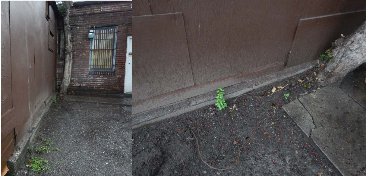
Photograph 3: Southern border of the Building Addition, facing east, showing wiring identified by the utility locator to be conductively grounded to the same location as the three pipes. The wiring led from the window behind the tree pictured, and continued below ground and potentially beneath the Building Addition.
