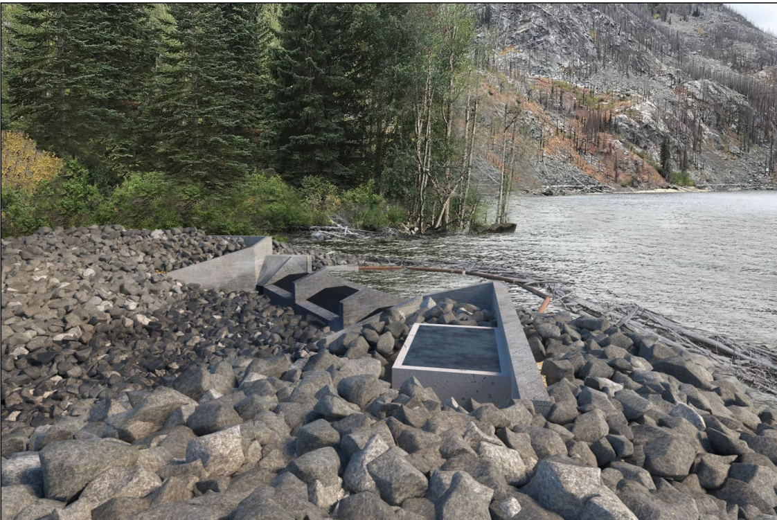
Figure 11-17b. Simulated view from KVP A of Alternative 1 with Gates in Lowered Position (water level 4,667 feet)
