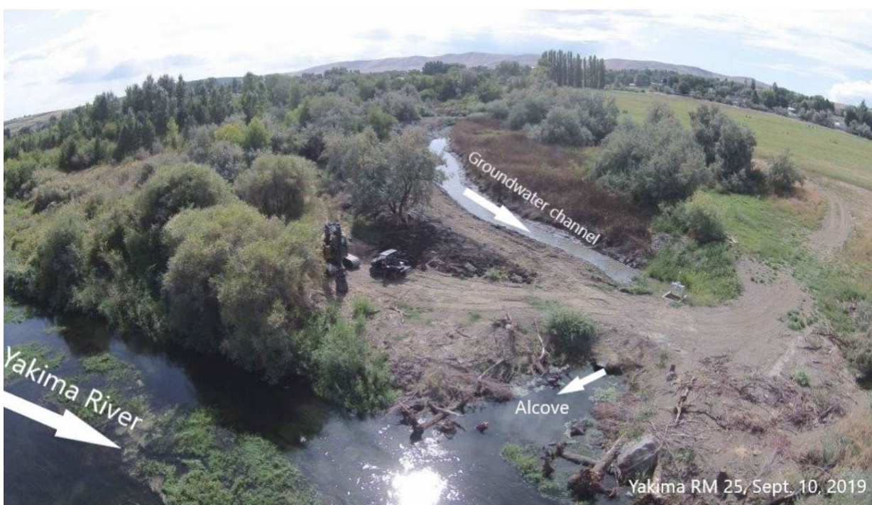
Figure 2. River Mile 25 Pilot Project for Thermal Refuge Enhancement. Photo shows enhanced groundwater channel, installed alcove and mainstem Lower Yakima River.
