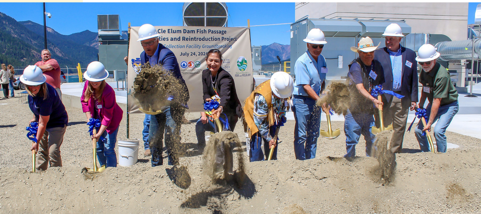
Yakima Basin Integrated Plan partners break ground on the upstream adult fish collection facility at Cle Elum Dam July 24, 2024. Pictured: Bureau of Reclamation PNW Regional Director Jennifer Carrington, Ecology Director Laura Watson, Governor Jay Inslee, Interior Secretary Deb Haaland, Yakama Nation Chairman Gerald Lewis, Roza Irrigation District Board Member Ric Valicoff, Leon Louis (Lower Similkameen Indian Band, Syilx Nation), Department of Agriculture Director Derek Sandison, Department of Fish and Wildlife Commissioner Steve Parker. Credit: Yakima Basin Integrated Plan
