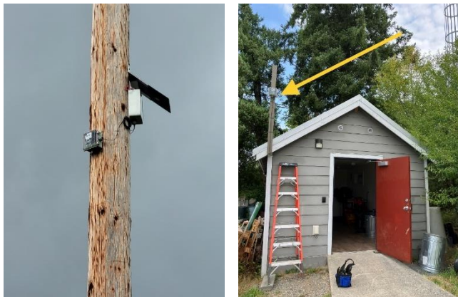
SensWA elevated on utility pole (left) and outbuilding (right).
