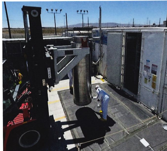
Workers remove a spent ion exchange column from the Tank-Side Cesium Removal System enclosure.
