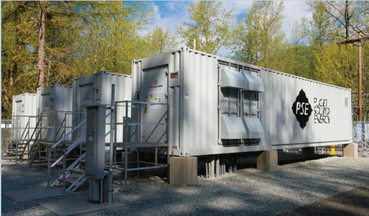
Example of a BESS interior
