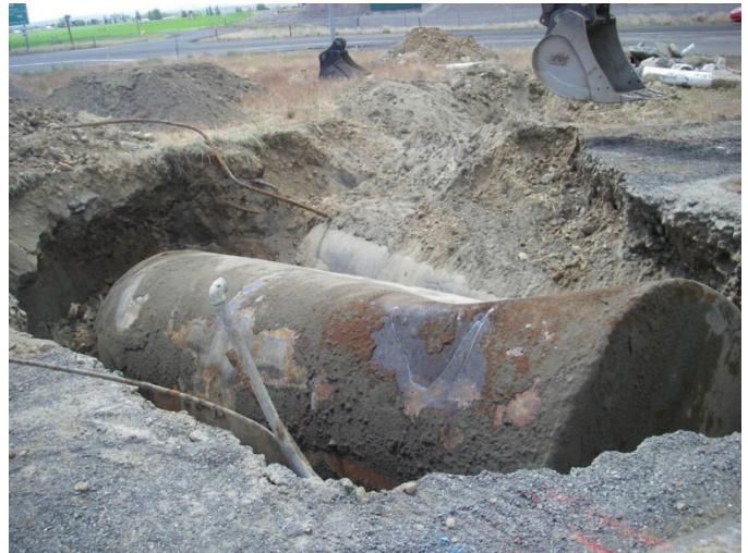
Underground storage tanks can be a potential source of contamination.
