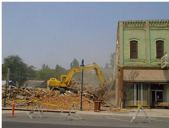
Figure 7. Demolishing the buildings on the site included abatement of lead- and asbestos-containing materials.
