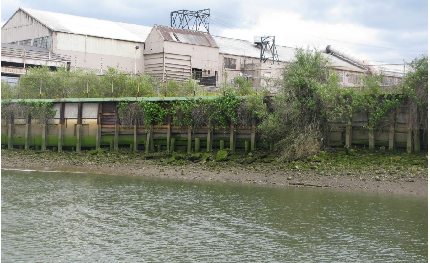
Port of Seattle's wooden bulkhead on the northern side of the Site.
