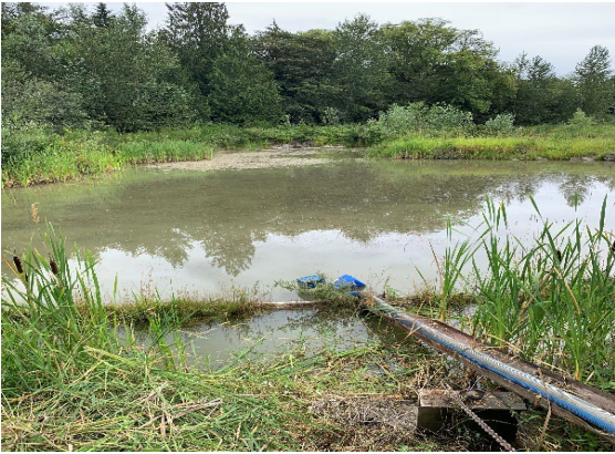
Infiltration pond for treated concrete wastewater.
