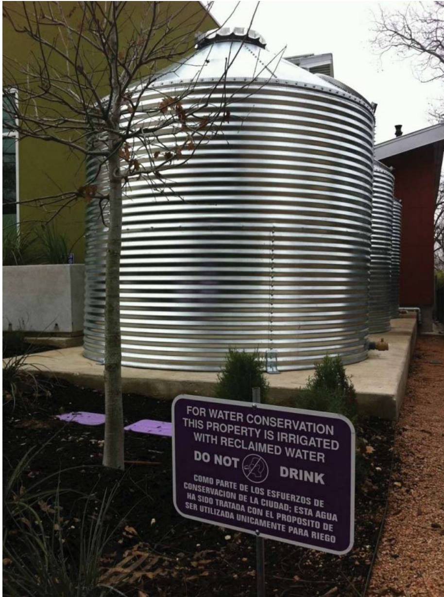
Figure 6.89: Cistern Used to Meet Irrigation Requirements
