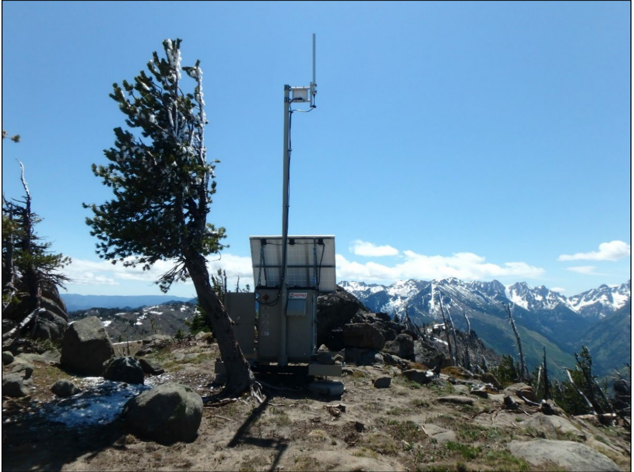
Figure 9. Forest Service Existing Repeater Station on Icicle Ridge
