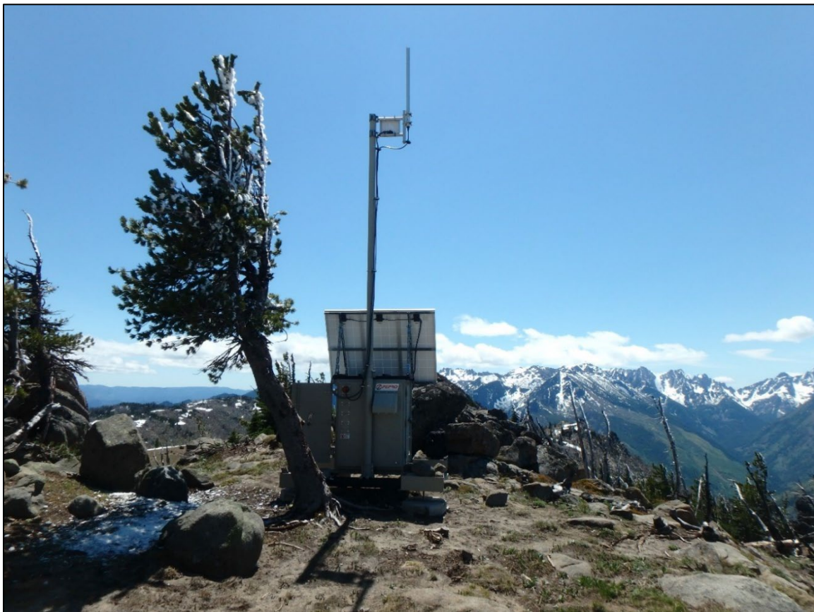
Figure 2-10. Forest Service Icicle Repeater Station
