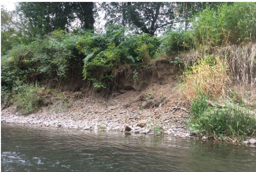
Figure 3. Evidence of toe erosion at bottom of riverbank
