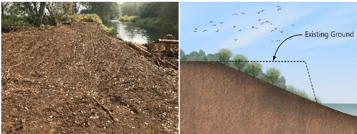
Figure 17. Sloping or removing fill Freshly excavated and seeded slope adjacent to Skookumchuck River. Photograph courtesy: Anchor QEA.
