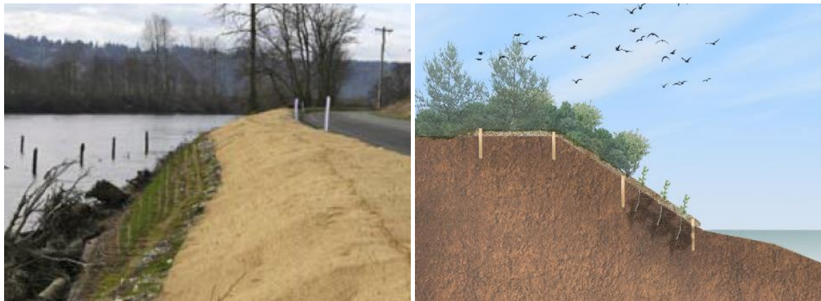
Figure 9. Erosion control blanket
