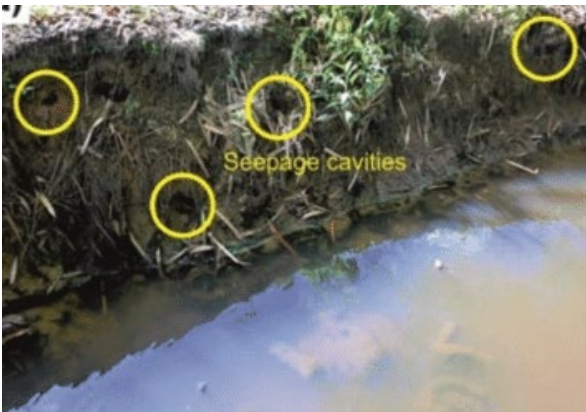
Figure 6. Seepage cavities observed along riverbank (yellow circles)
