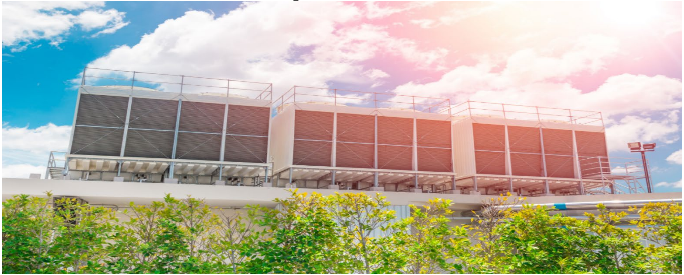
Figure 1. Large air-conditioning unit containing hydrofluorocarbons (HFCs)
