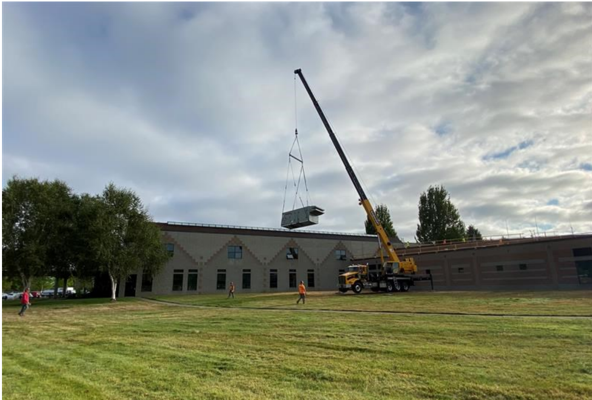
Figure 9: Construction on the Chief Leschi School to improve heating and ventilation. CCA funding enabled this project to give cleaner air to the school's students while also electrifying the old system which reduced emissions. Reducing on-site fossil fuel burning can improve air quality. Photo credit to OSPI.
