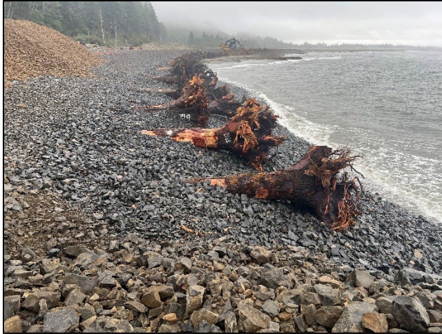
Figure 12. Work at State Route 105 to address significant coastal erosion. The completed project includes a wave-absorbing barrier that mimics a natural cobble beach. Credit – Washington State Department of Transportation
