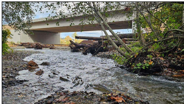
Figure 3. A new State Route 3 bridge over Chico Creek in Kitsap County replaced an undersized culvert, which restored fish passage, addressed chronic erosion of the road embankment, and is more resilient to precipitation and tidal events. Credit – Washington State Department of Transportation
