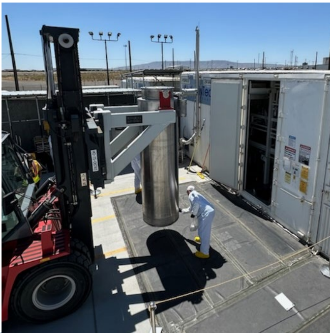
Workers remove a spent ion exchange column from the Tank Side Cesium Removal System enclosure.
