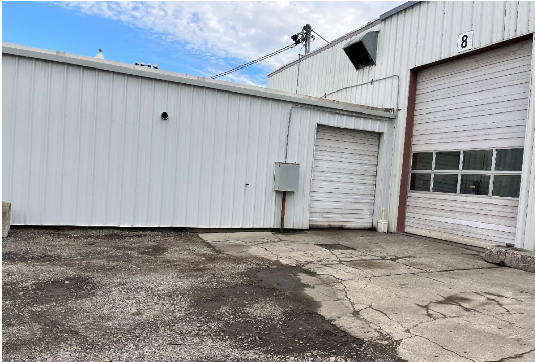
Photo 3: Area of remaining contamination near former steam room — from the west
