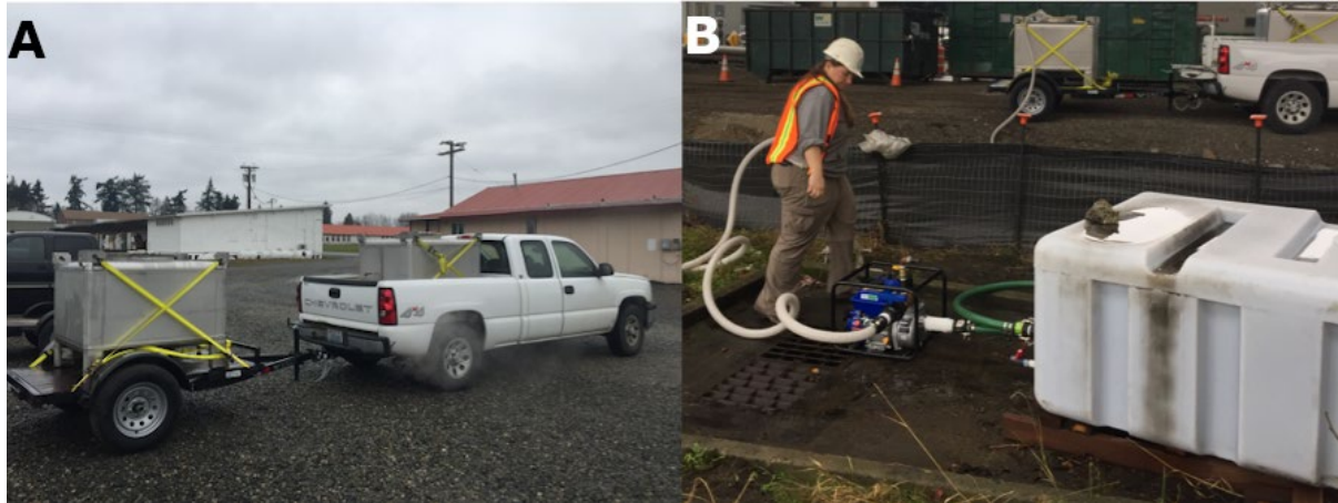
Figure 4. Stormwater runoff collection process. A) Stainless-steel transportation tanks at the WSU-Puyallup campus ready to transfer stormwater from the collection site. B) Stormwater runoff pumped from the polyethylene collection tanks to the stainless-steel transportation tanks using a gas-powered pump and food-grade hosing.
