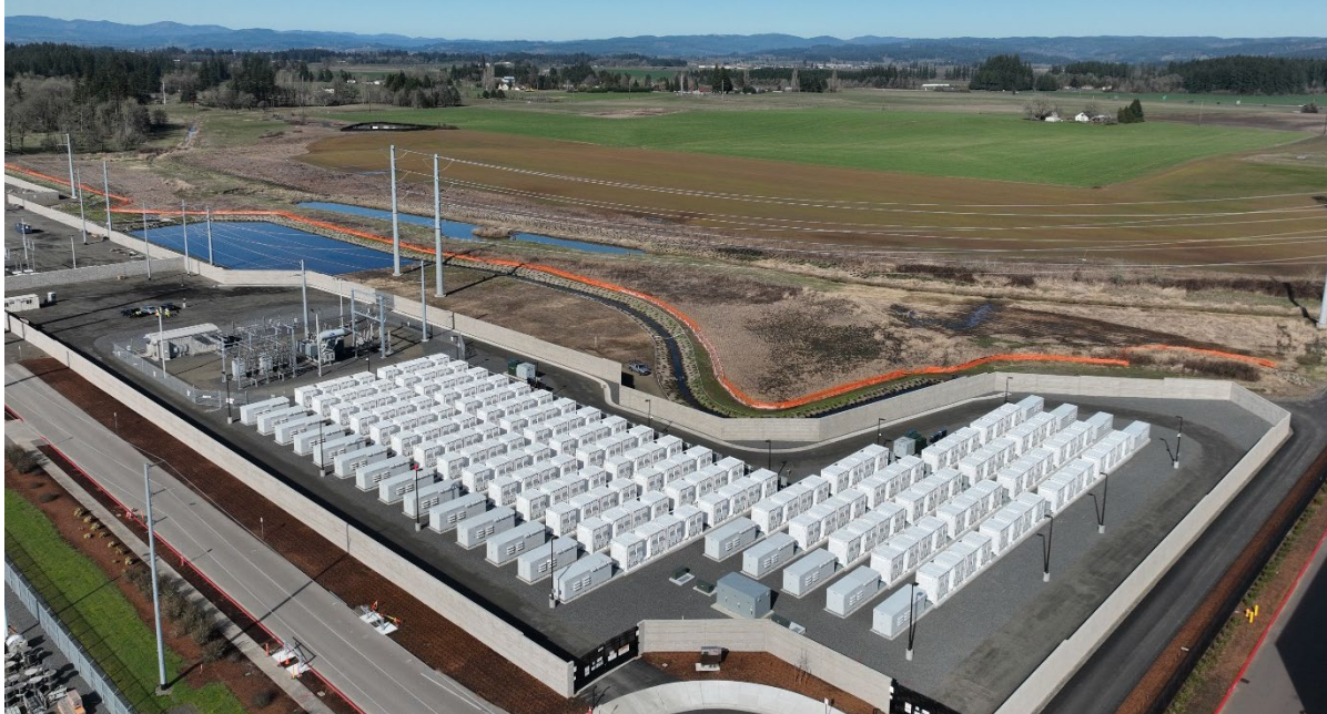
Figure 3. Example of utility-scale BESS facility (photo from Portland General Electric)
