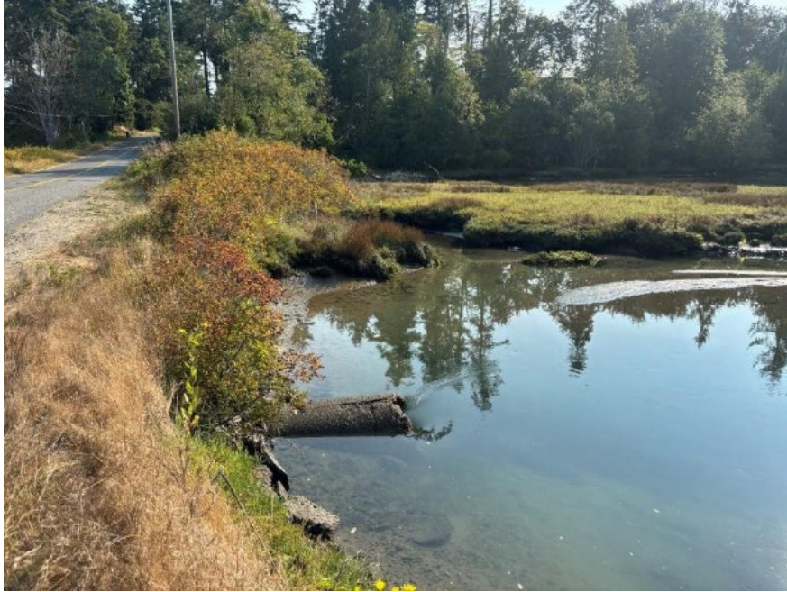
Figure 10: Road and undersized culvert impeding fish passage at Harper Estuary in Kitsap County. (Photo credit: Kitsap County Department of Community Development.)
