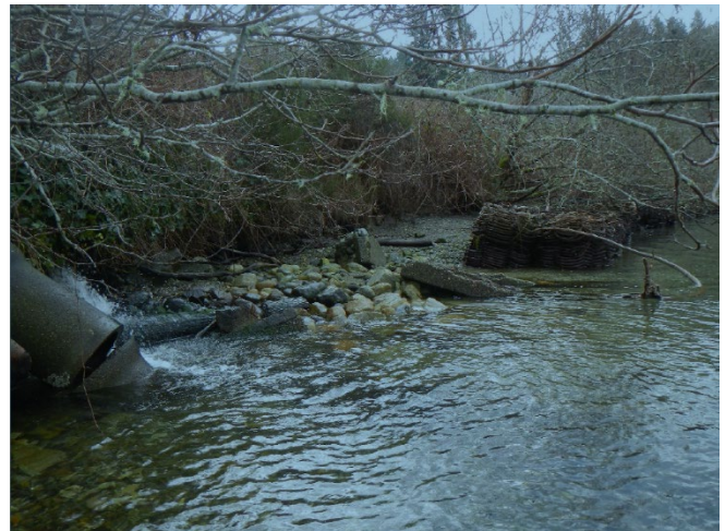
Figure 9: Undersized culvert and metal torpedo netting along the marine shoreline at Floyd's Cove on McNeil Island (Photo credit: WDFW).
