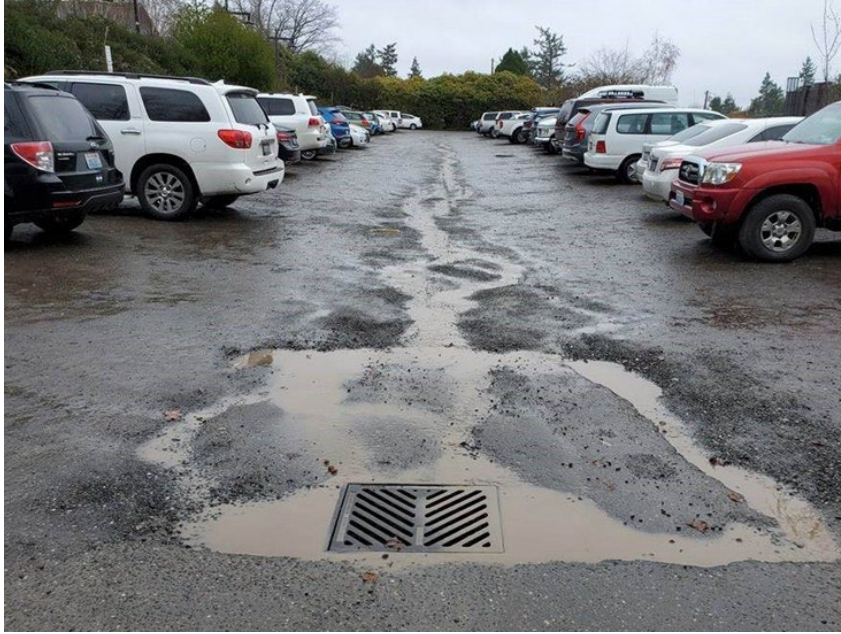
4 Untreated stormwater carries pollutants directly into local waterways. Photo by: City of Bainbridge Island.
