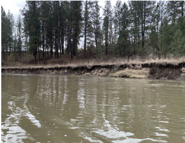
5 Eroding streambanks carry sediment and pollutants directly into the river. Photo by: Spokane Conservation District.
