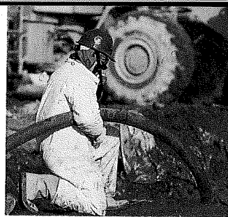
A cleanup worker prepares Atochem North America's site for treatment of contaminated groundwater. The project is part of a voluntary action under an Ecology consent agreement.
