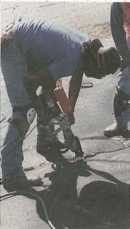
A worker seals a seam on the synthetic liner covering the Midway Landfill in Kent. The liner is one of several technologies used to solve pollution problems at the site.
