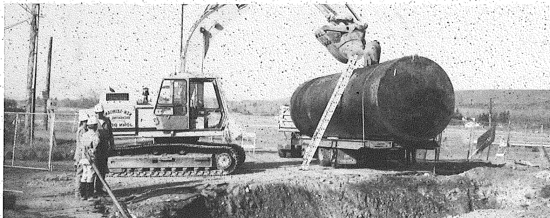
Workers remove an underground storage tank from the Bingo Fuel Stop site in Thorp, near Ellensburg.
