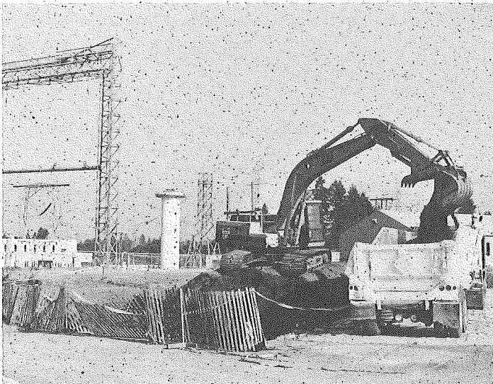
Contaminated soil is loaded into a plastic-lined trailer at the Bonneville Power Administration Ross Complex in Vancouver.
