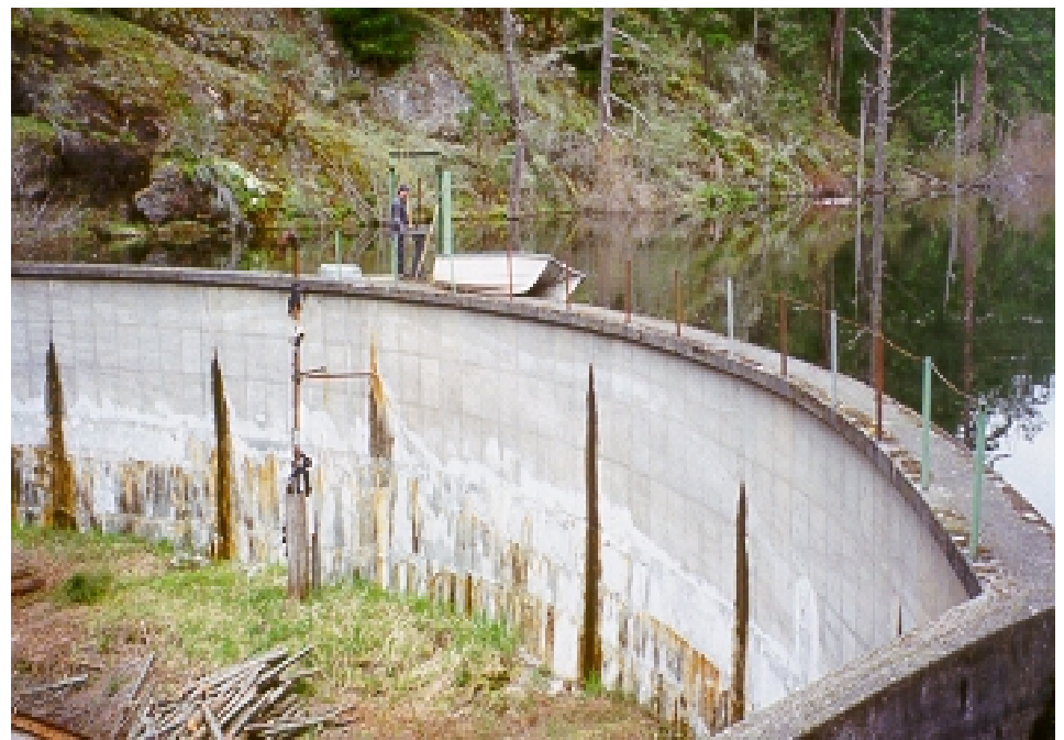
Typical aging concrete dam. Ecology is stepping up inspections of small dams located above areas where population is increasing. Photo: Doug Johnson
