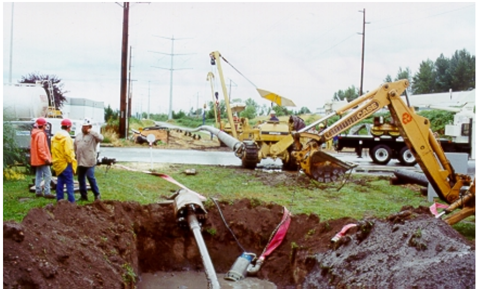
Workers line up a pipeline segment for direction drilling under the Green River. Photo: Paul Substis
