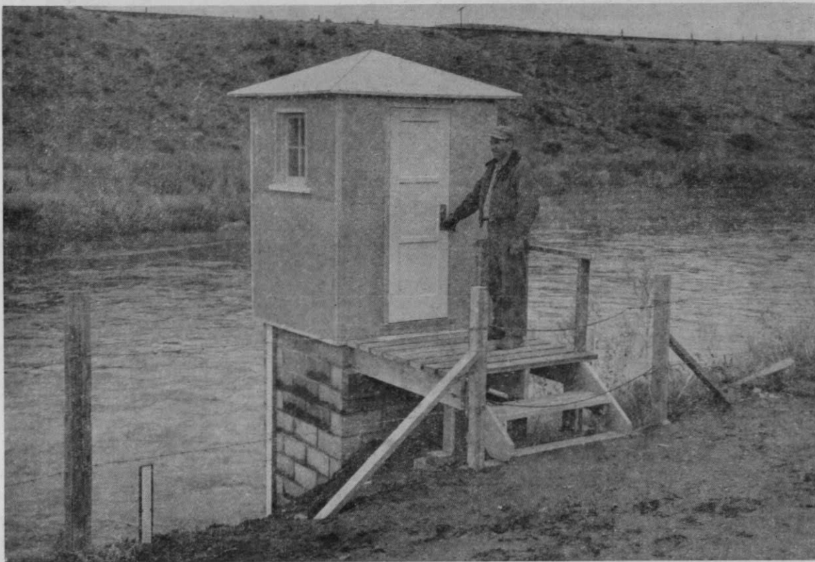
Figure 23. Concrete block well and aluminum-covered gage house on Walla Walla River near Touchet. Note outside vertical staff reference gage in two sections.
