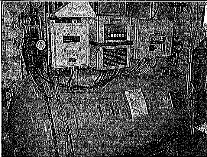
PHOTO #:15 DATE: SEPTEMBER 18, 2009 TAKEN BY: MARK HENDERSON FILE No.: IMG_019 DESCRIPTION: OWS - FACET SYSTEM
