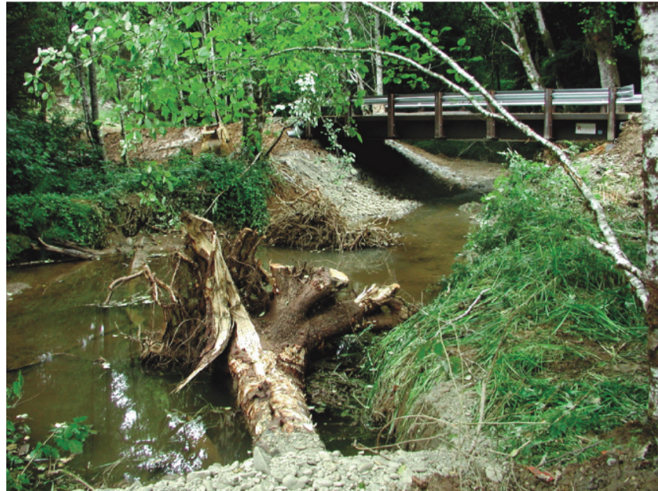
Before: a failing culvert. After: a bridge and fish-friendly woody debris are placed in a small, privately owned forest in the Chehalis area (Department of Natural Resources photos)
