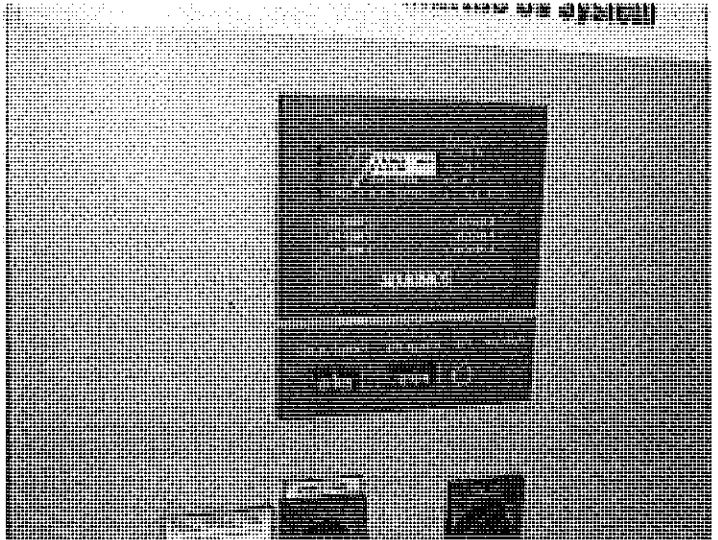
PHOTO #:22 DATE: SEPTEMBER 12, 2010 TAKEN BY: AMY JANKOWIAK FILE No.:P9120031 DESCRIPTION: UV SYSTEM ELECTRONICS
