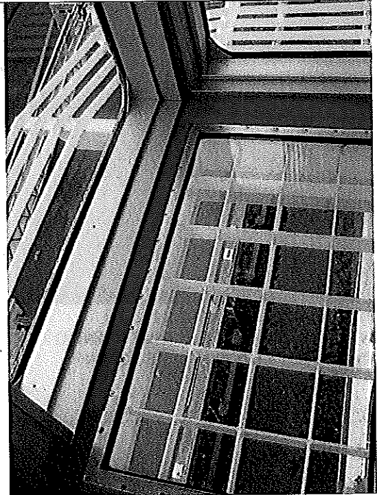
PHOTO #:04 DATE: SEPTEMBER 24, 2010 TAKEN BY: AMY JANKOWIAK FILE No.:P9240004 DESCRIPTION: BRIDGE - VIEW BELOW
