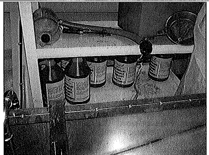
PHOTO #:16 DATE: SEPTEMBER 12, 2010 TAKEN BY: AMY JANKOWIAK FILE No.:P9120024 DESCRIPTION: MEMBRANE FILTERS CLEANING CHEMICALS (MEMBRANE CLEANER ORGANIC ACID)
