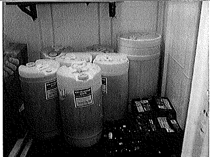
PHOTO #:08 DATE: JULY 31, 2010 TAKEN BY: KEVIN C. FITZPATRICK FILE No.: P7310012 DESCRIPTION: HAZARDOUS WASTE STORAGE
