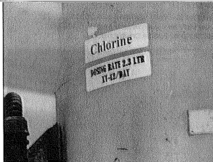
PHOTO #:23 DATE: SEPTEMBER 24, 2010 TAKEN BY: AMY JANKOWIAK FILE No.:P9240029 DESCRIPTION: MSD CHLORINE DOSING
