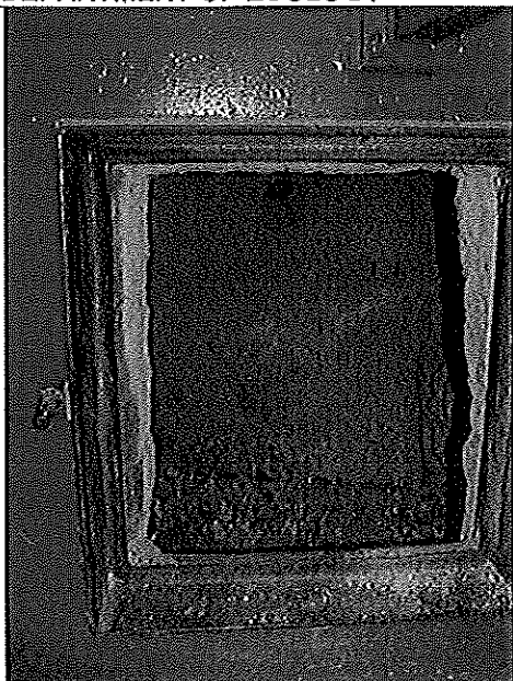
PHOTO #:25 DATE: JUNE 18, 2010 TAKEN BY: AMY JANKOWIAK FILE No.:P6180056 DESCRIPTION: INSIDE OF INCINERATOR
