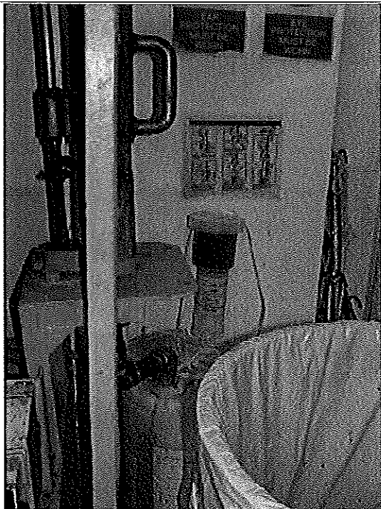
PHOTO #:21 DATE: JULY 6, 2010 TAKEN BY: AMY JANKOWIAK FILE No.:P7060081 DESCRIPTION: AEROSOL WASTE COLLECTION SYSTEM
