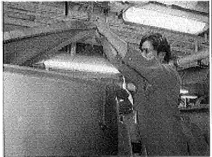
PHOTO #:36 DATE: AUGUST 29, 2010 TAKEN BY: LORI LEVANDER FILE No.: P8290140 DESCRIPTION: FLOTATION TANK
