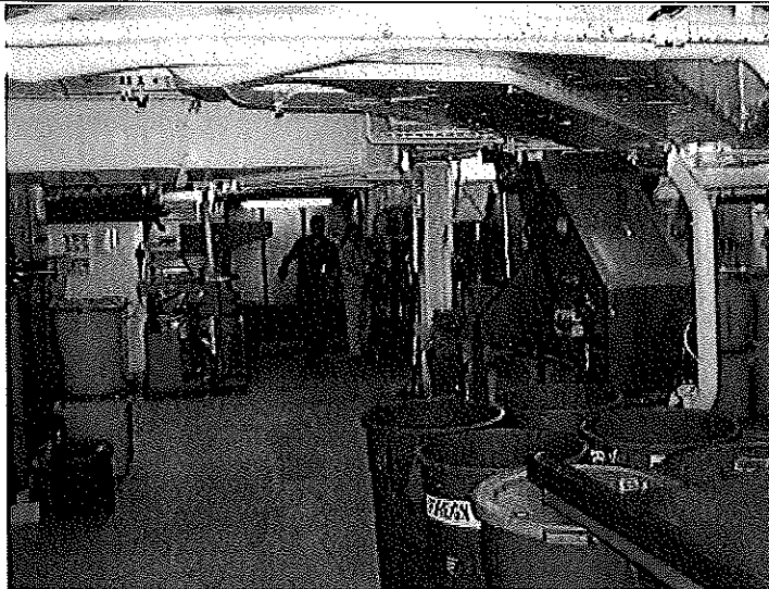
PHOTO #:07 DATE: JULY 31, 2010 TAKEN BY: KEVIN C. FITZPATRICK FILE No.: P7310011 DESCRIPTION: GARBAGE/RECYCLING ROOM
