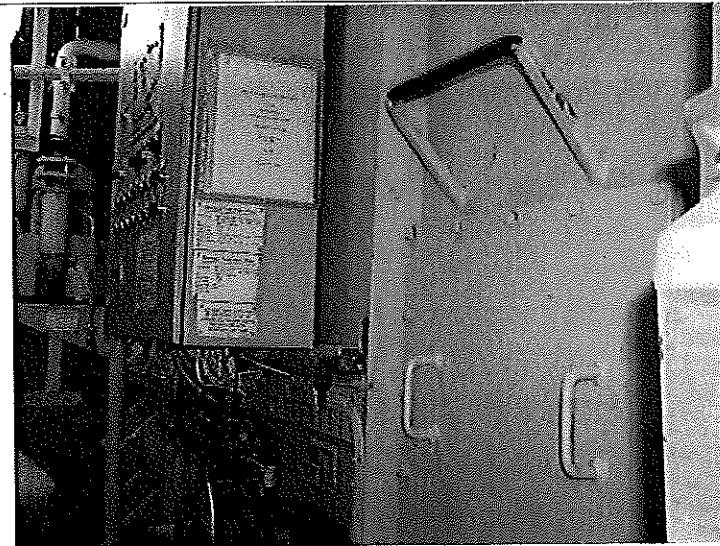
PHOTO #:04 DATE: JULY 6, 2010 TAKEN BY: AMY JANKOWIAK FILE No.: P7060063 DESCRIPTION: BLACK WATER TREATMENT SYSTEM (TRITON) (1 OF 4)
