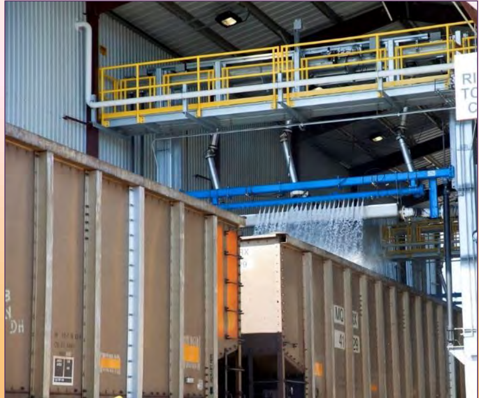
Rail car spray station in Pasco Photo UTC
