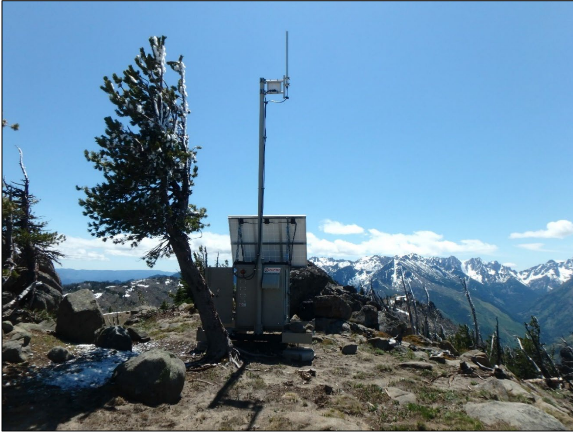
Figure 9. Forest Service Icicle Repeater Station
