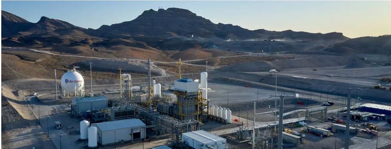
Figure 7. Steam-methane reforming and liquid storage facility – Air Liquide – Apex, NV
