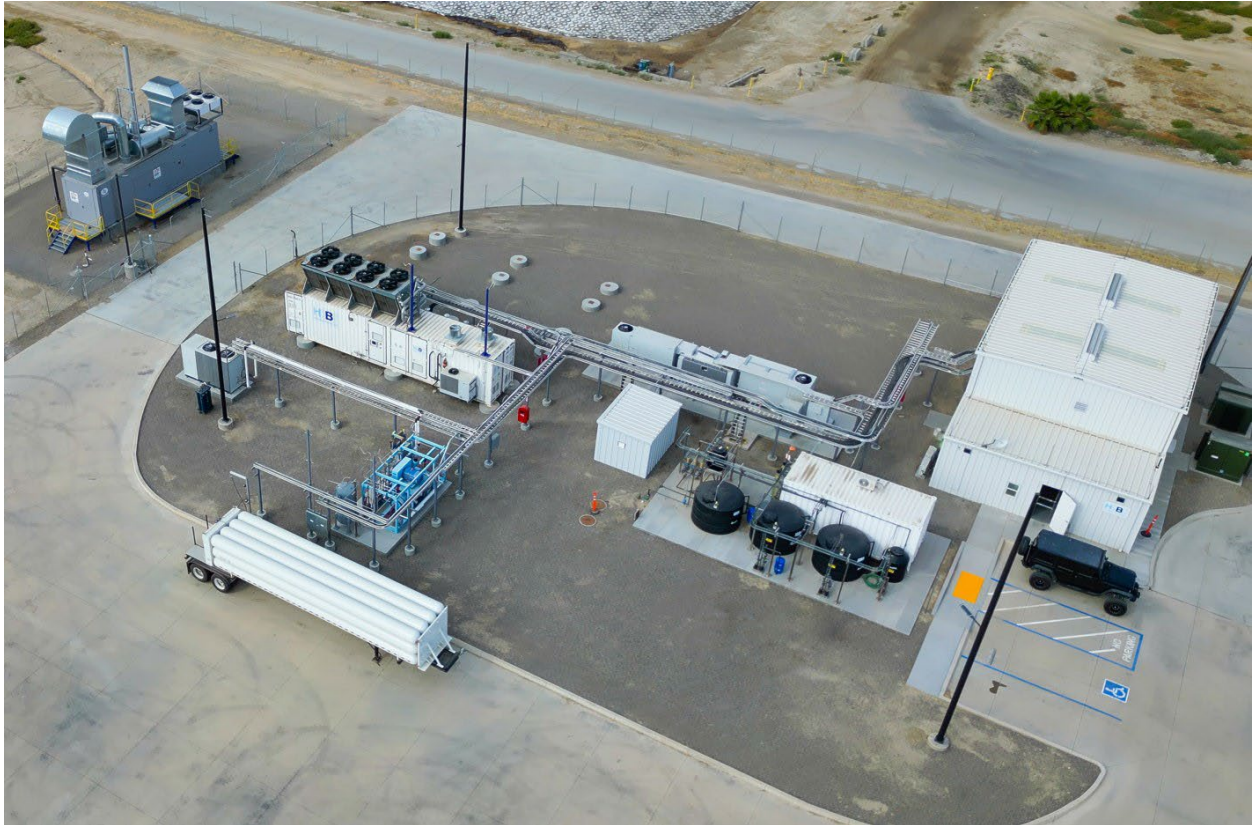
Figure 9. Electrolysis facility – H2B2 SoHyCal – Fresno, CA
