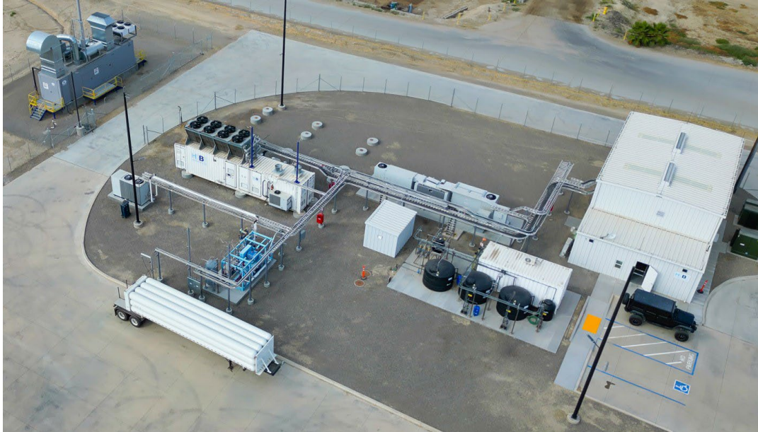
Figure S-4. Electrolysis facility – H2B2 SoHyCal – Fresno, CA Source: H2B2 Electrolysis Technologies 2023
