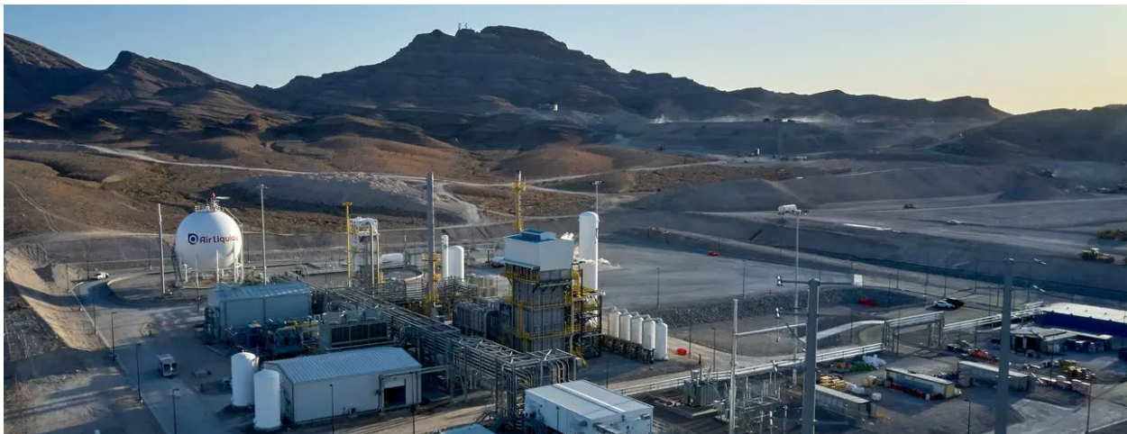
Figure S-5. Steam methane reforming and liquid storage facility – Air Liquide – Apex, NV Source: Air Liquide 2022
