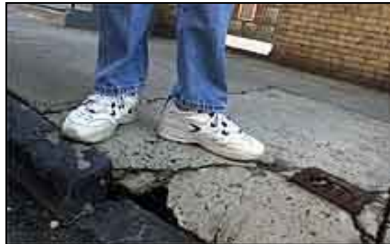
Figure 1: Pavement damage due to pipe leak
